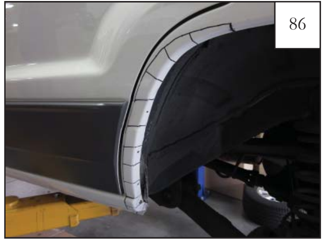
Mark vehicle for cutting: Make marks from inner wheel well to line drawn in previous steps about 2" apart as shown in picture. Make marks closer together around tight corners and style lines.
