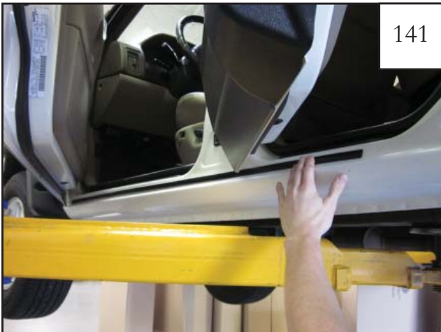
Remove tape liner from molding (GP1-0020) and starting at front hole, install molding along rocker area to cover holes in sheet metal.
